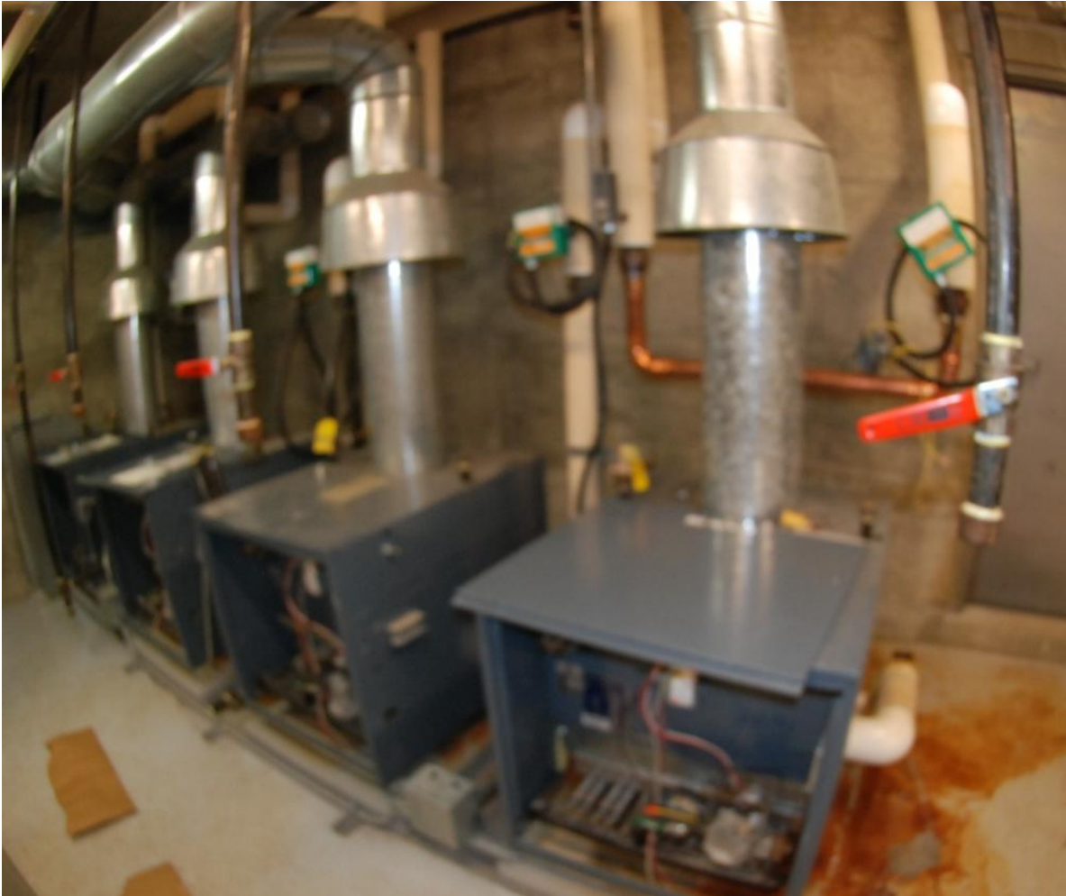
Natural draft boilers
